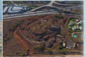
Mass grading of approximately 27,000 CY and 20,000 CY of embankment with grading of approximately 12 acres
