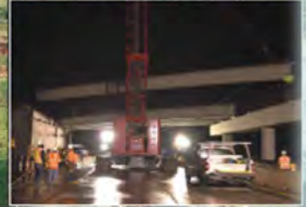
Waikea Overpass was constructed at night requiring closure of H-1. Traffic detours provided to maintain access to Waikoloa Coast (H-1, facing eastbound).
